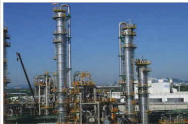
Chemical Lines, Gas Lines
